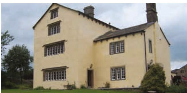
Cement render removed and replaced with hydraulic lime render to restore breathability and flexibility.
